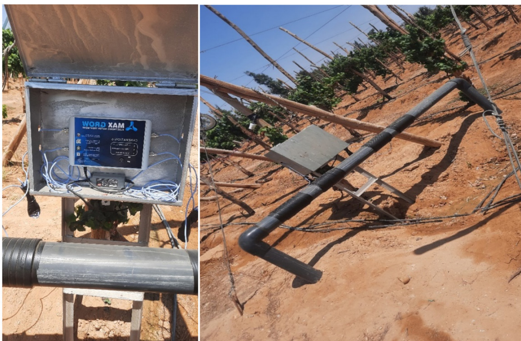
Figure 2: The Max Grow water treatment technology system used in EL-Wafrah Vineyard
